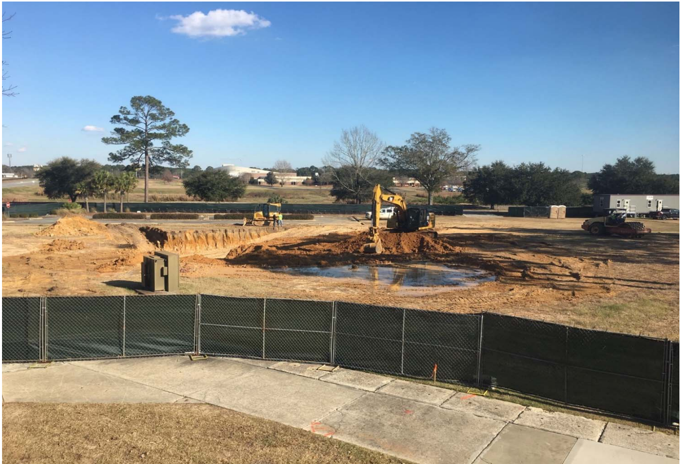
Update 1-28-2019 - Foundation work for the new Fine Arts building on Sweetheart Circle begins
